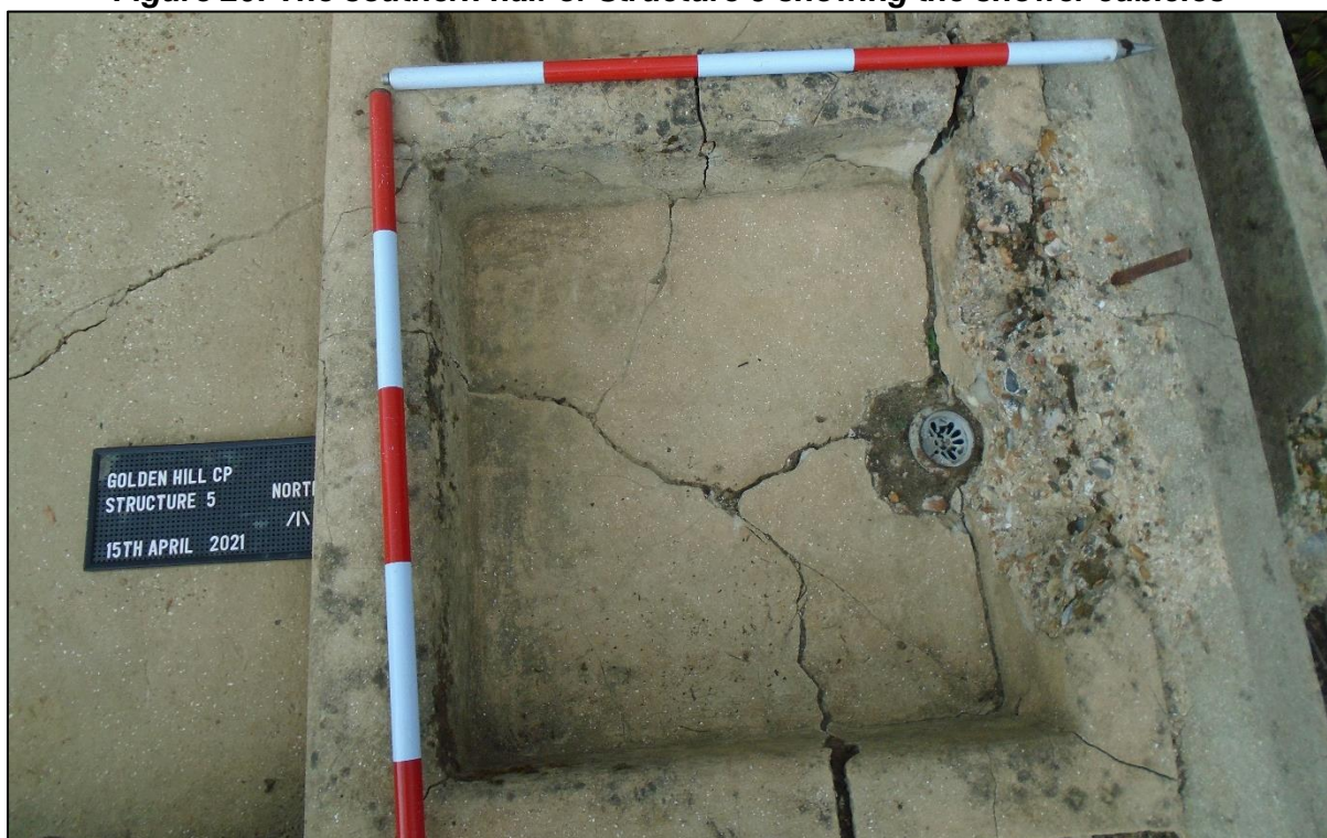
Figure 21: One of the drain strainers within one of the shower cubicles in Structure 5
