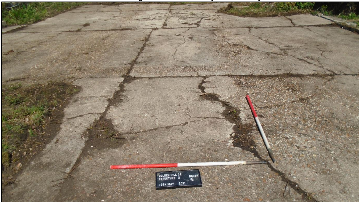
Figure 13: Wear patterns in central level of Structure 2
